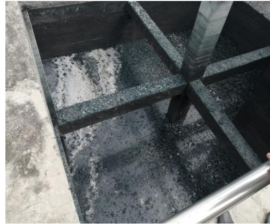
Sludge collection tanks
