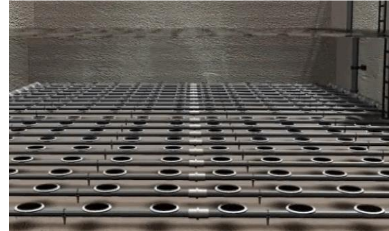
Fine bubble diffused aerators
