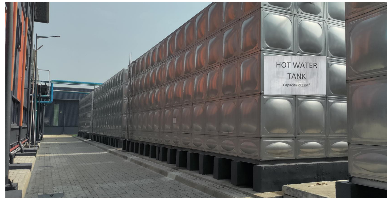
Storage tank for hot water, cooling water. Copyright: Mohammad Abbas Uddin
