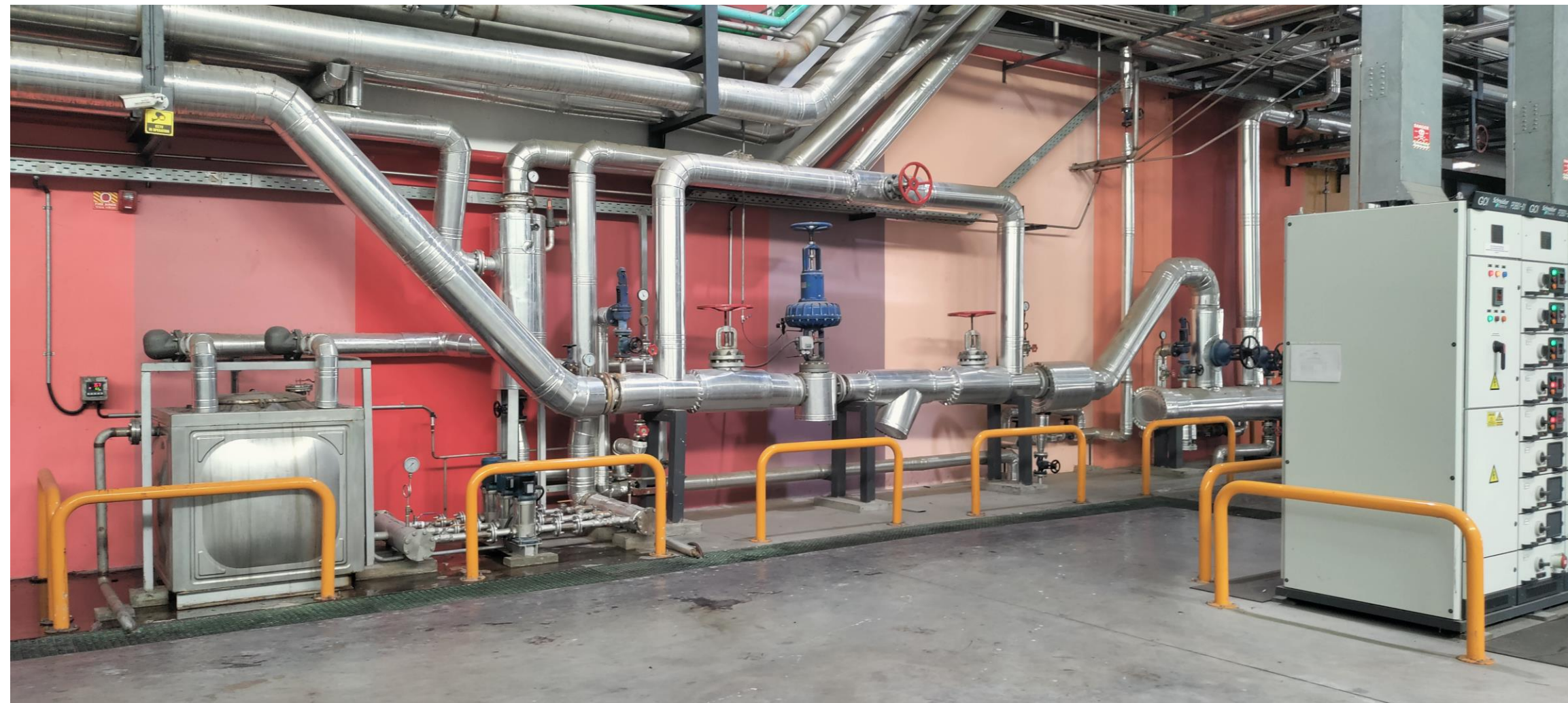
Condensate Recovery system. Copyright: Mohammad Abbas Uddin
