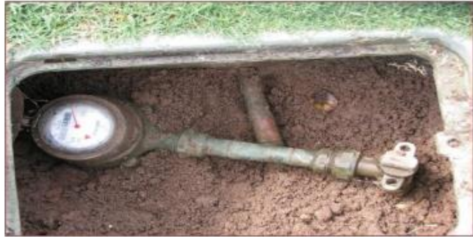
Pipe used to partially bypass water meter.
