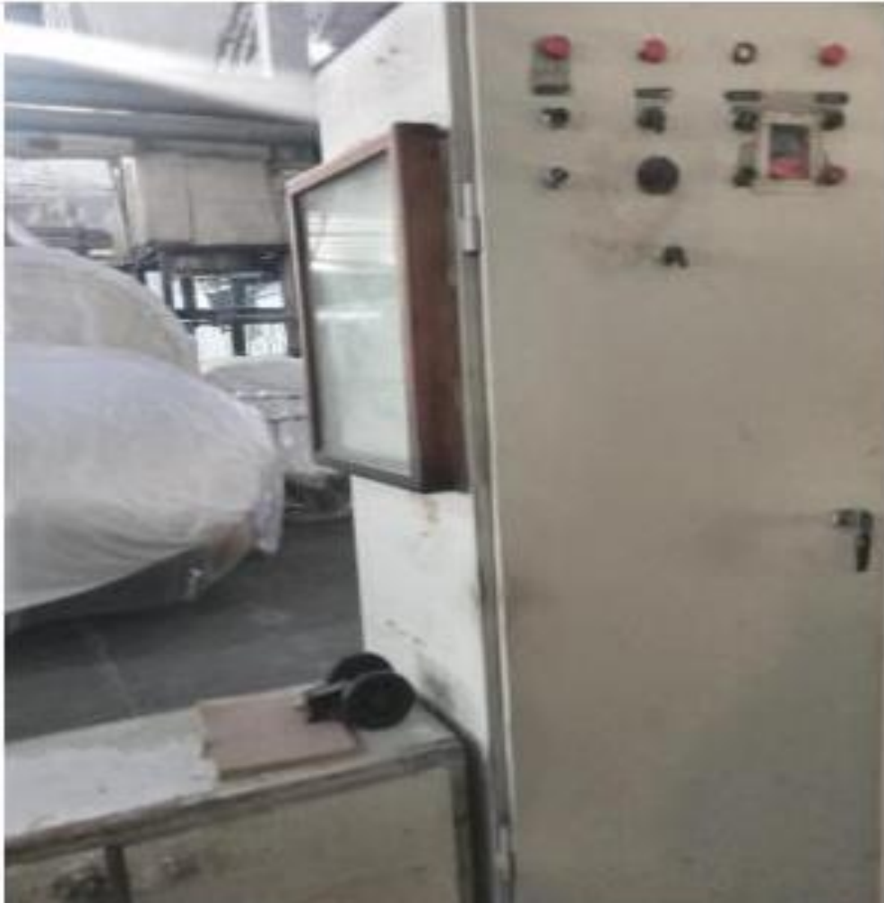
Absence of electric hazard symbols from DB board
