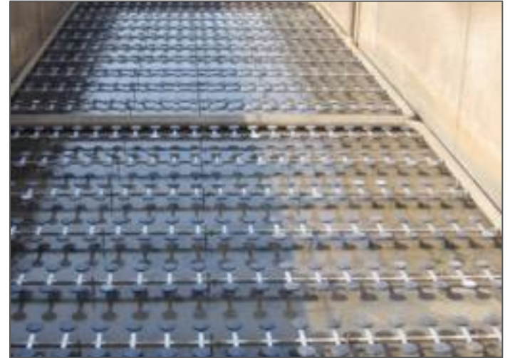
Diffusers in equalization tank
