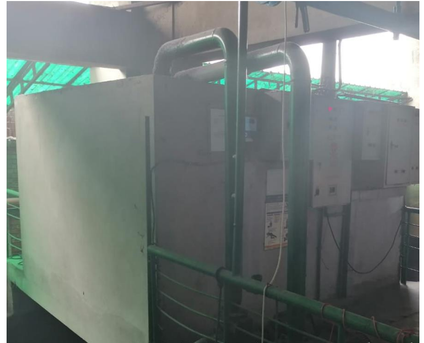
Cooling system at aeration tank inlet
