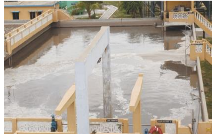
Equalization tank with jet aeration
