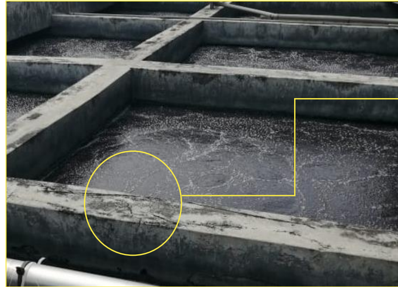
Slippery platform without handrail
