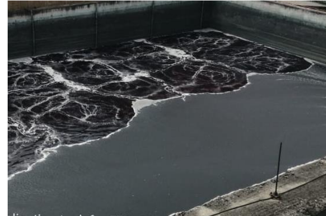
Aeration tank with dead spots: Indication of blocked diffusers
