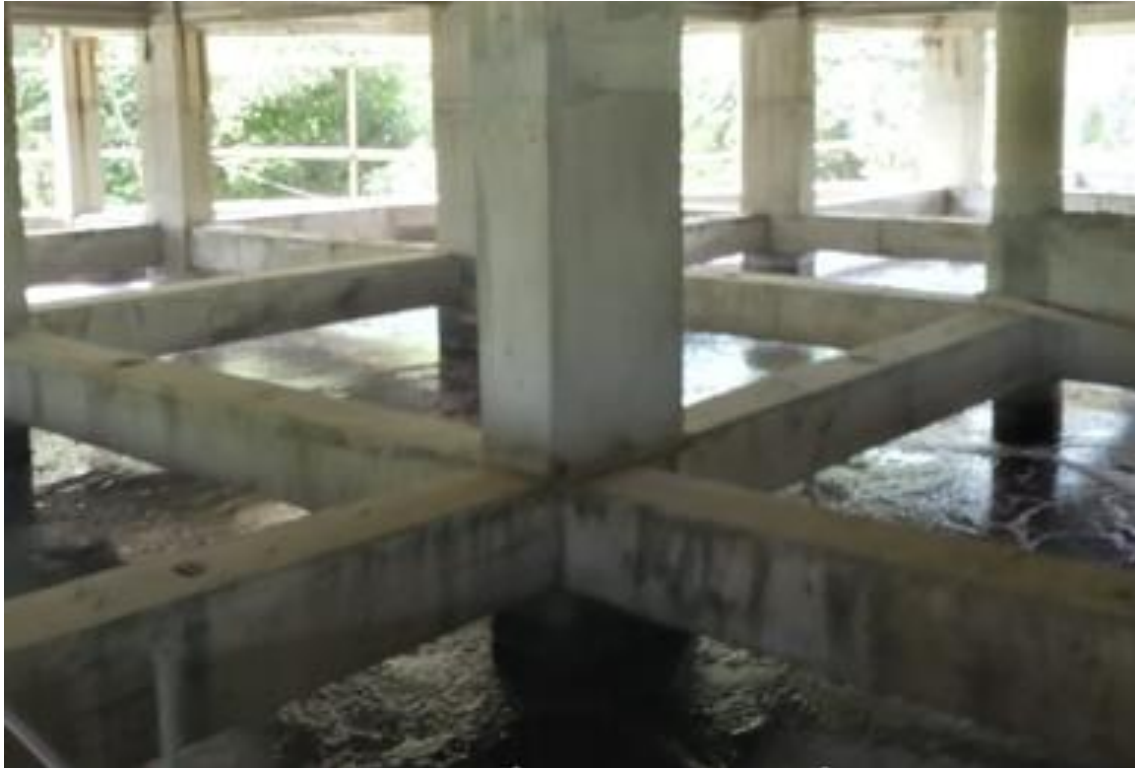
Aeration tank constructed as double decker to save space.
