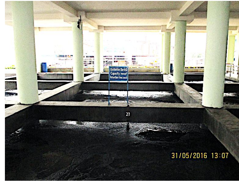
Conventional aeration tank
