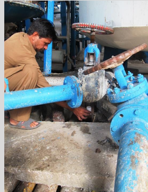
Attending to leaking valves and pipe connections of a chemical dosing system
