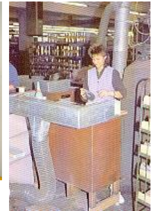
Use of local exhaust ventilation in glue application in shoe factory, Photo. AUVA
