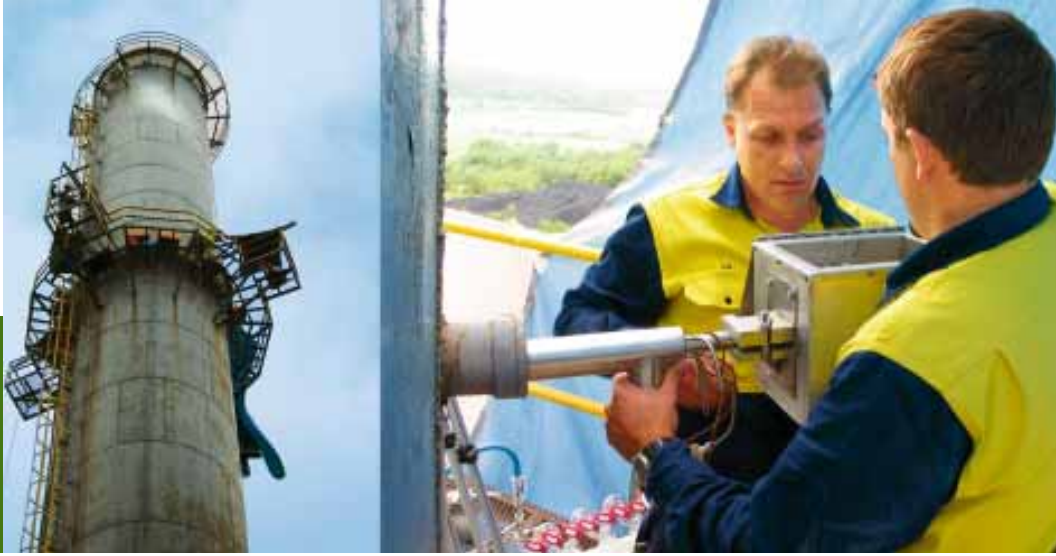
Stack with the monitoring platform and the adjustment of the probe into the kiln
