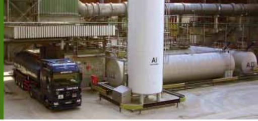
Storage and dosing of waste
