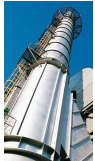
Stack with monitoring platform
