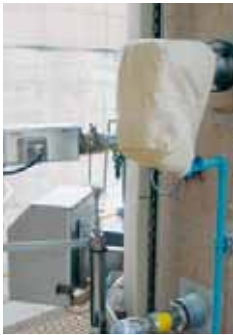
Continuous emission monitoring equipment in place
