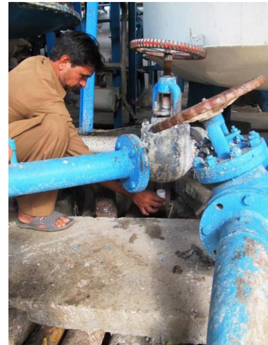
Attending to leaking valves and pipe connections of a chemical dosing system
