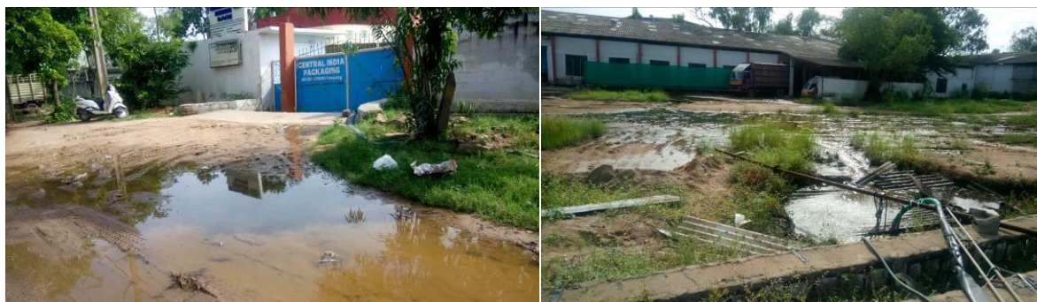
FIGURE 4: WATER LOGGING IN THE INDUSTRY AFTER 3 DAYS OF HEAVY RAINFALL
