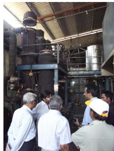
Image no. 21: Installed Caustic Recovery Unit by Textile Industry [Source: GIZ-IGEP and GCPC team]
