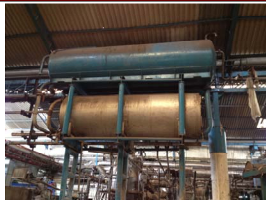
Image no. 25: Hot Water Generation & Storage Tank to Supply Hot Water to Jigger Machines [Source: GIZ-IGEP and GCPC team]
