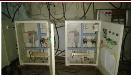
Image no. 28: Installed VFD for Jet Dyeing Machine Pumps
