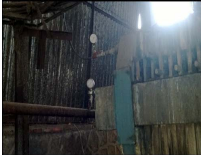
Image 30: Filter Press with Pressure Regulating Device [Source: GIZ-IGEP & GCPC Team]
